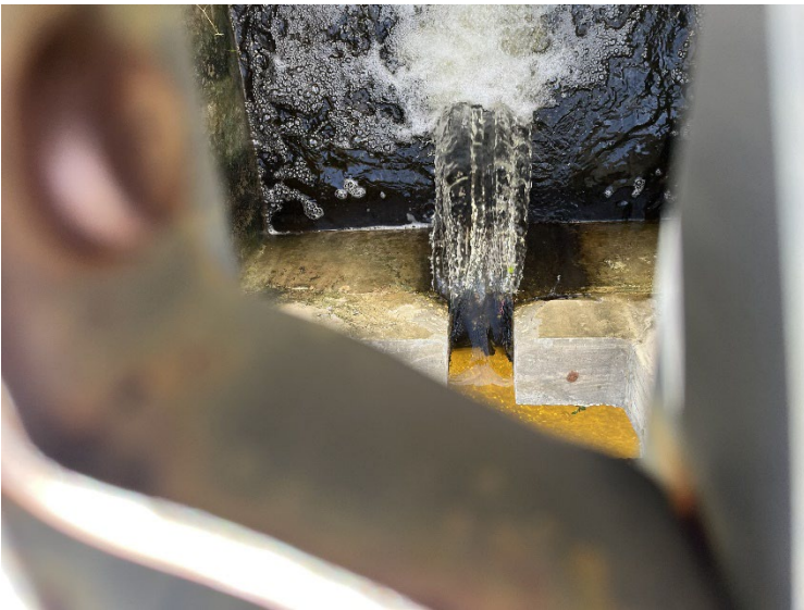
P-2 Weir clear/functional.
